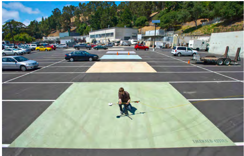
Jordan Woods of the Berkeley Lab Heat Island group takes measurements of new cool pavement coating using an albedometer. (Source: Lawrence Berkeley National Laboratory)
